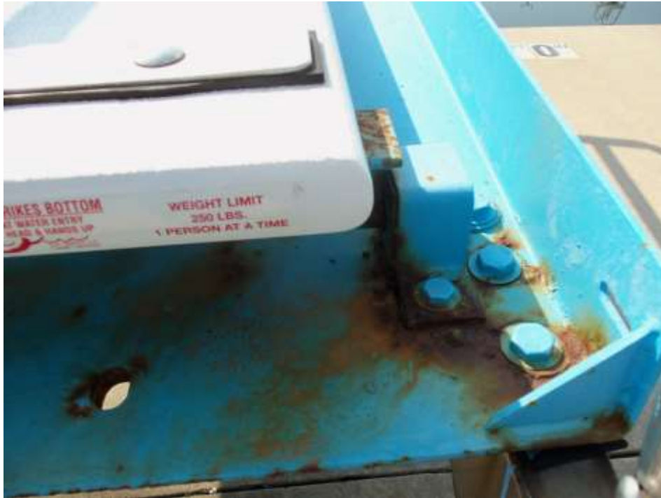
Diving Board Stand Requires Repair
