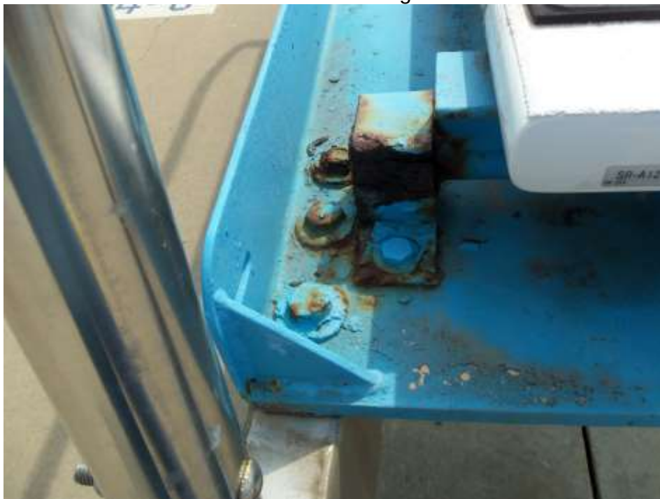
Diving Board Stand Requires Repair
