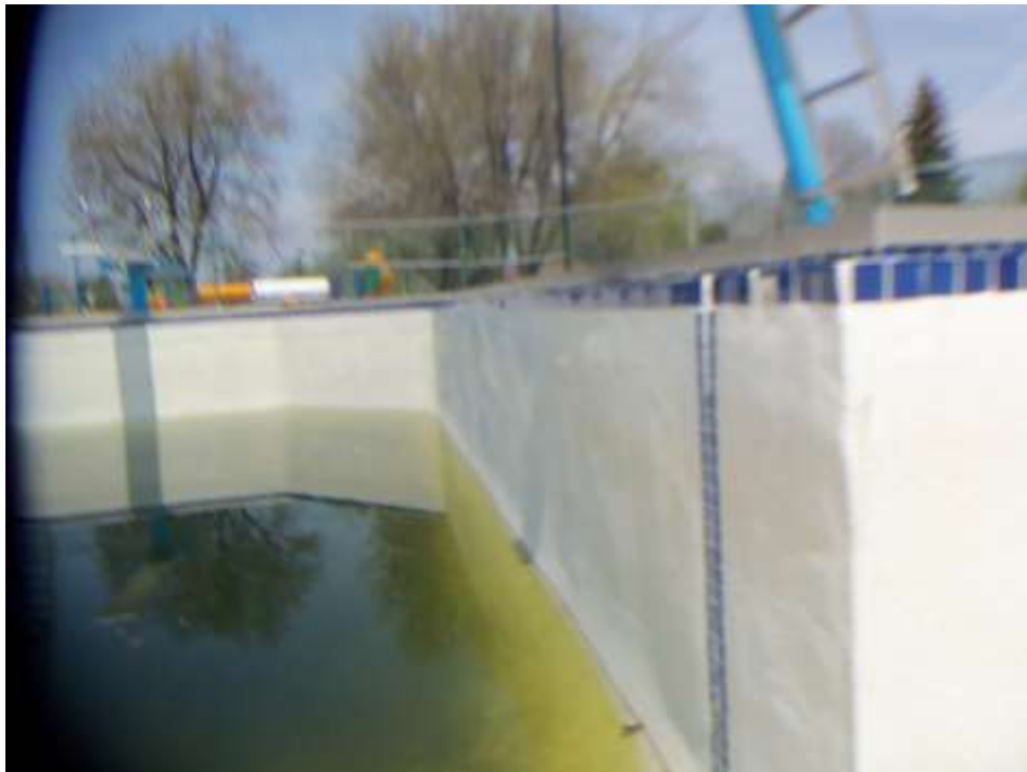
Pool Finish Failure
