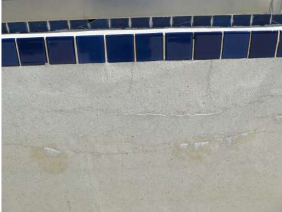
Pool Finish Failure
