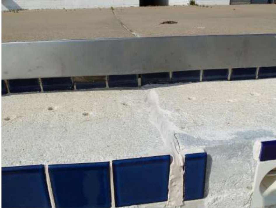
Expansion Joint Failure
