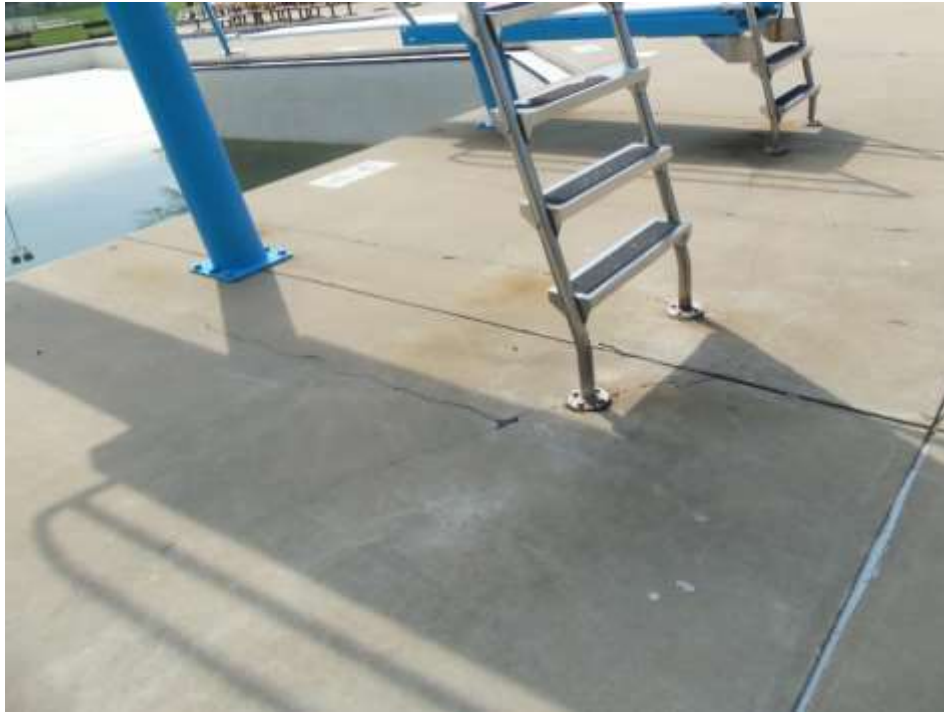
Deck Cracks at Diving Board
