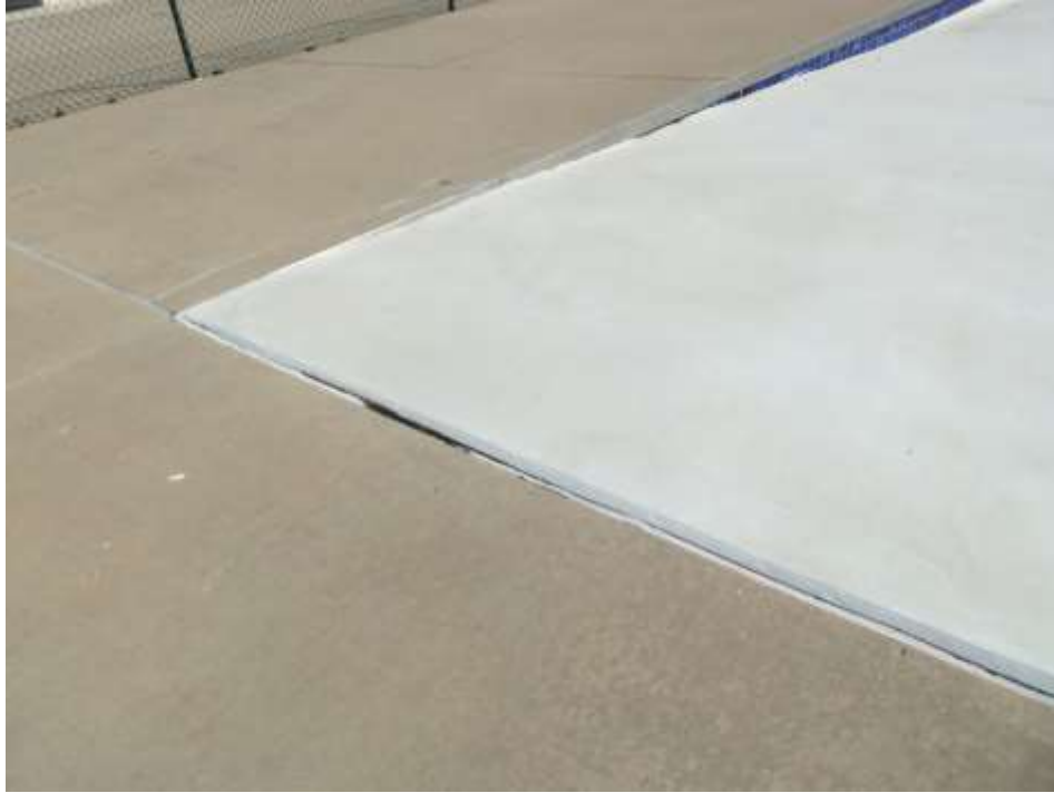
Tripping Hazard at Wading Pool
