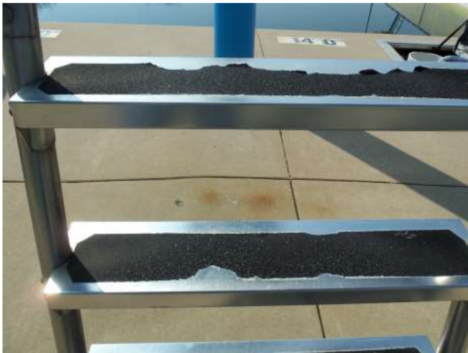
Diving Board Ladder Steps Are Slippery
