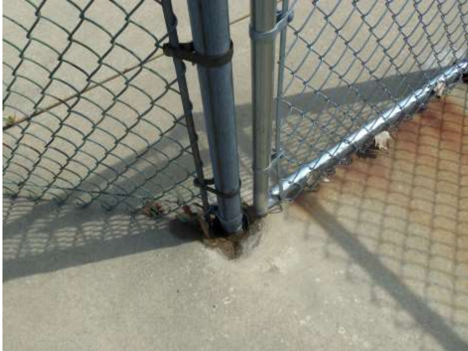
Corrosion at Barrier
