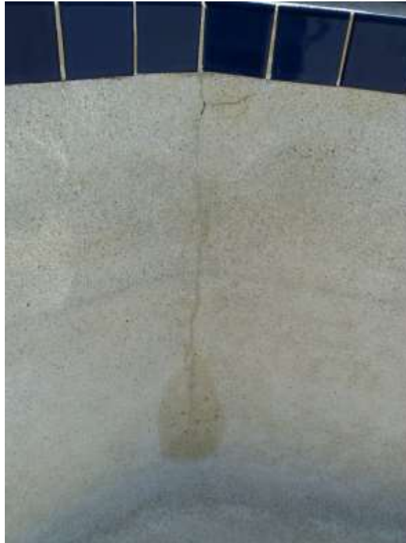
Pool Finish Failure
