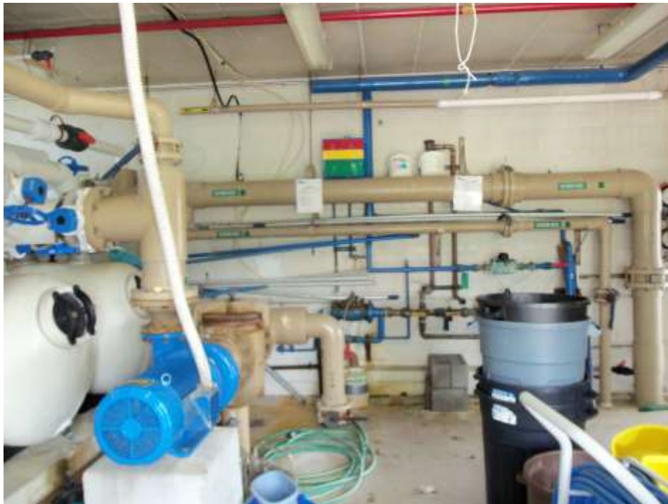
Filtration Pump and Strainer
