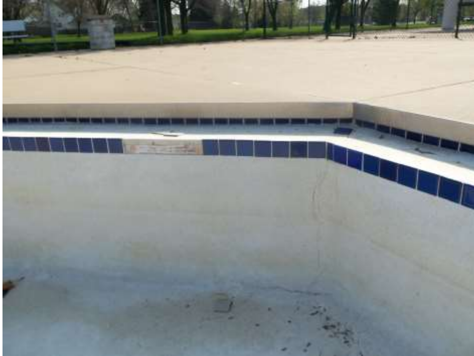
3"x3" Pool Wall Tile Failure
