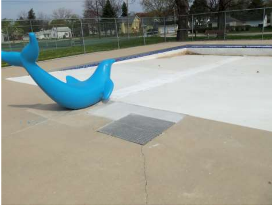
Wading Pool pipe was recently replaced. The Seal water does not work.
