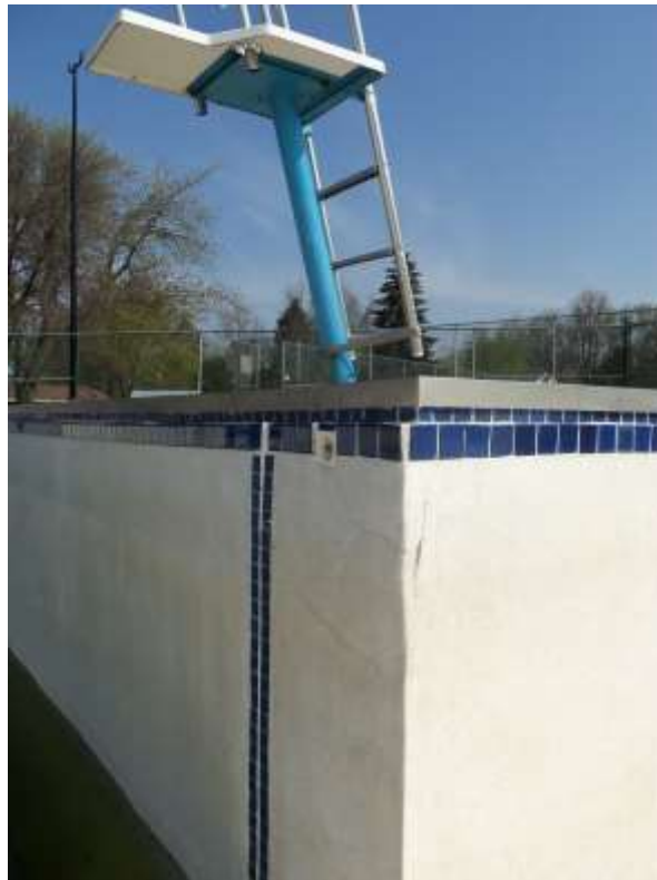
Pool Finish Failure
