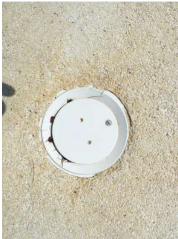
Cracked Floor Inlet Fitting
