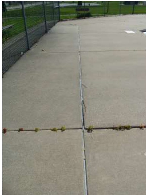
Deck Joints Require Repair
