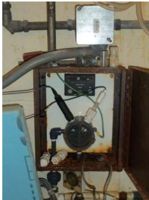
Pool Chemical Controller Probes
