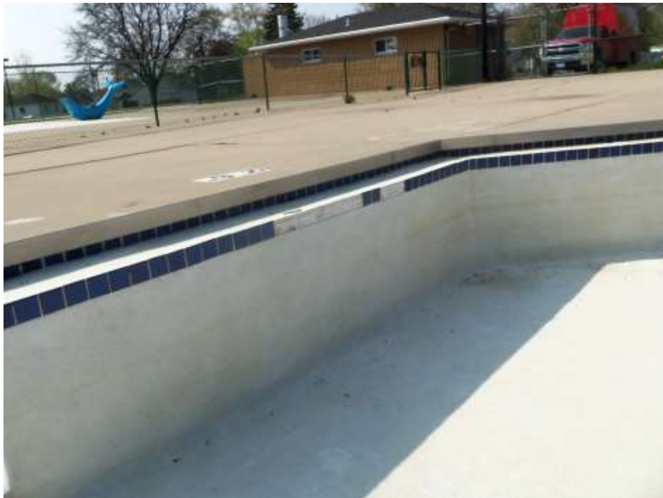
3"x3" Pool Wall Tile Failure
