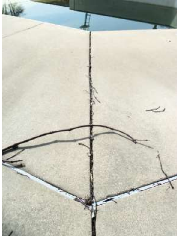
Deck Joints Require Repair
