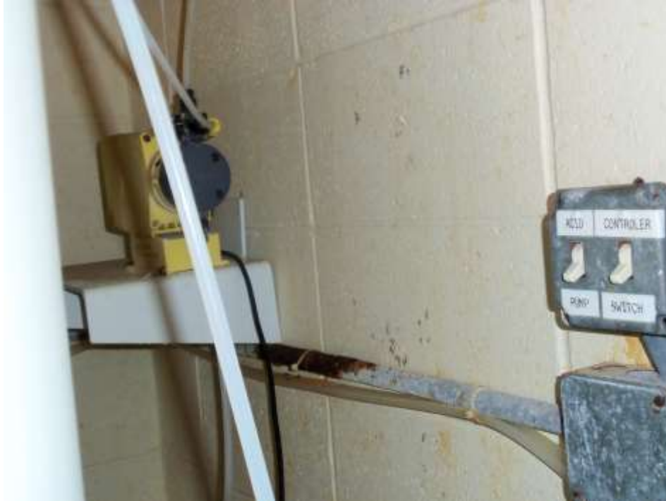
Pool LMI Acid Pump
