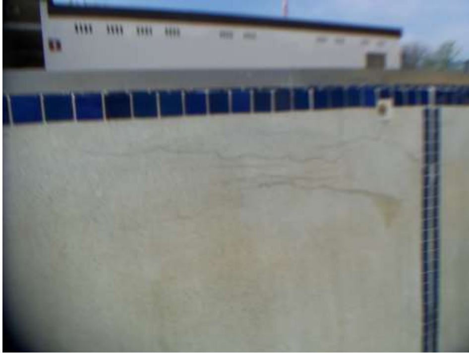
Pool Finish Failure
