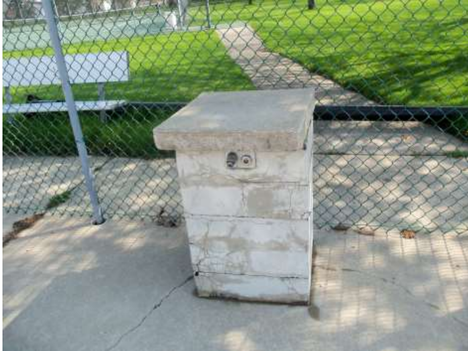
Hose Bibb Requires Repair
