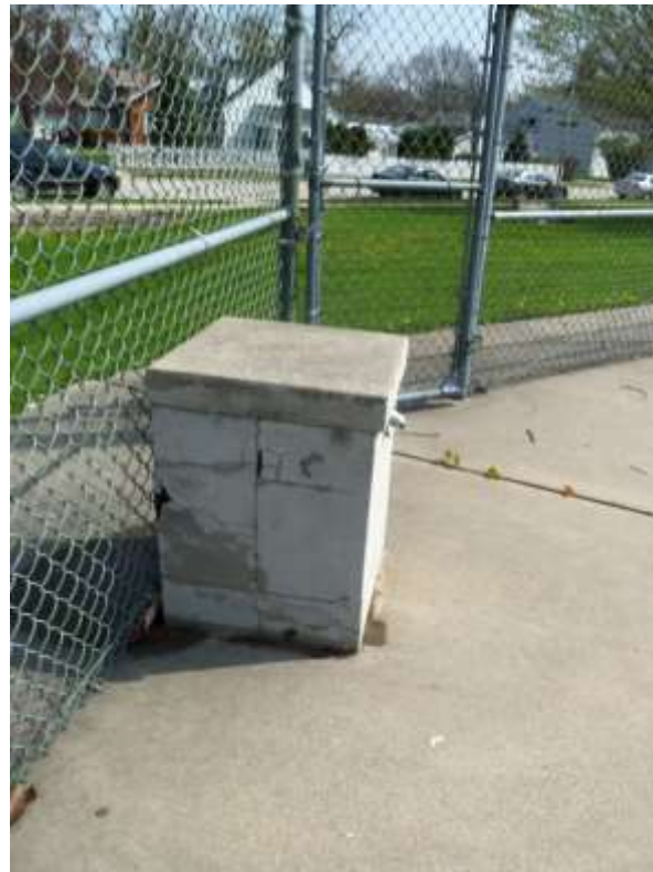
Hose Bibb Requires Repair
