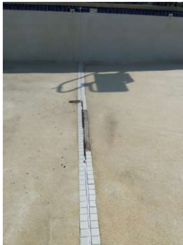
Expansion Joint Failure
