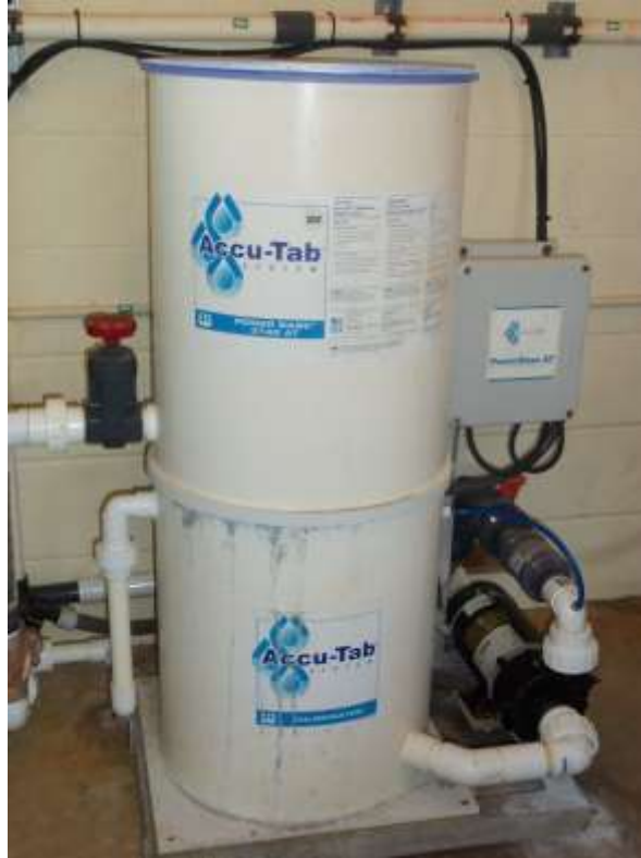
Pool Chlorine Feeder
