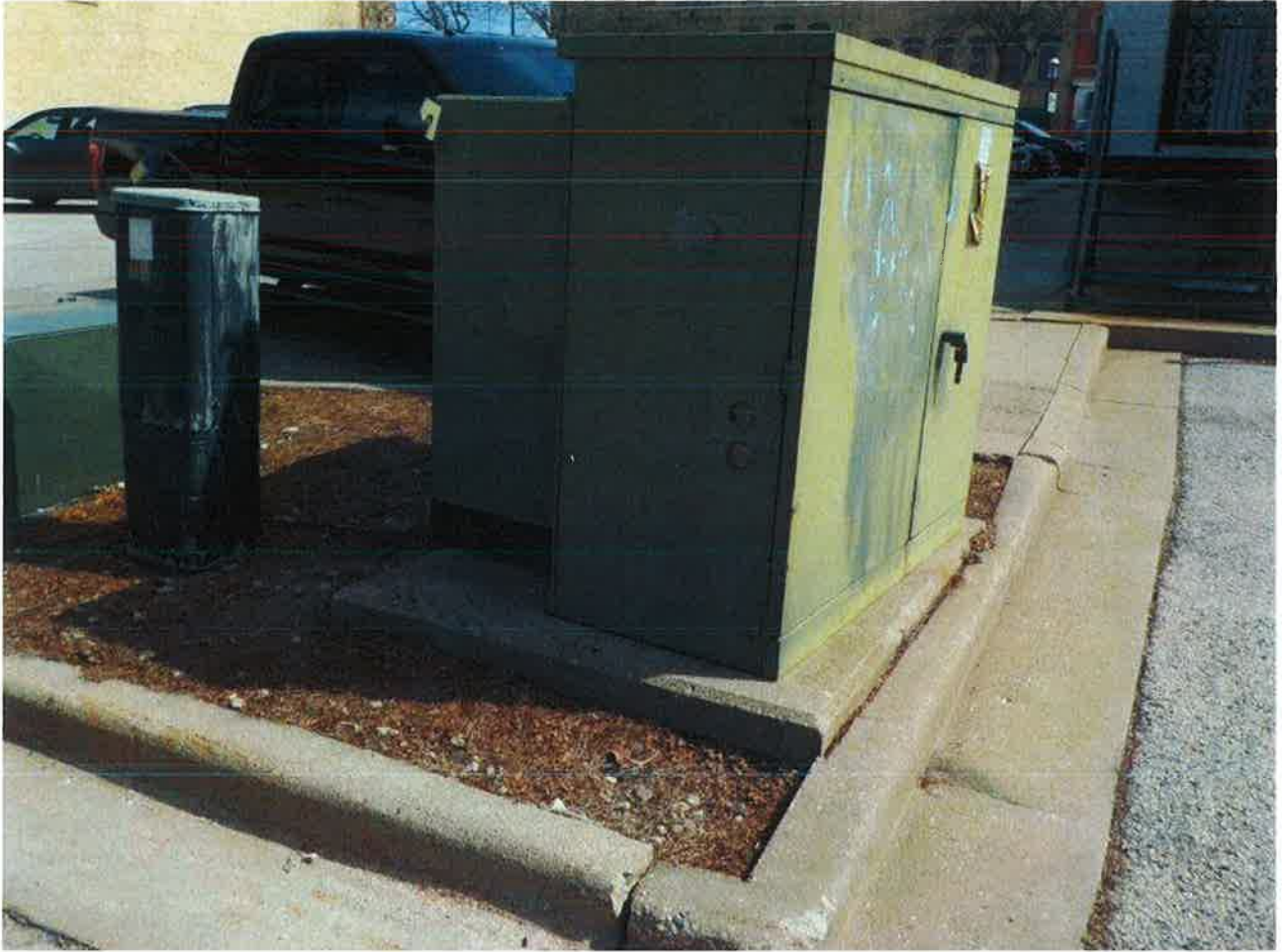
Pad mounted transformer along south property line.
