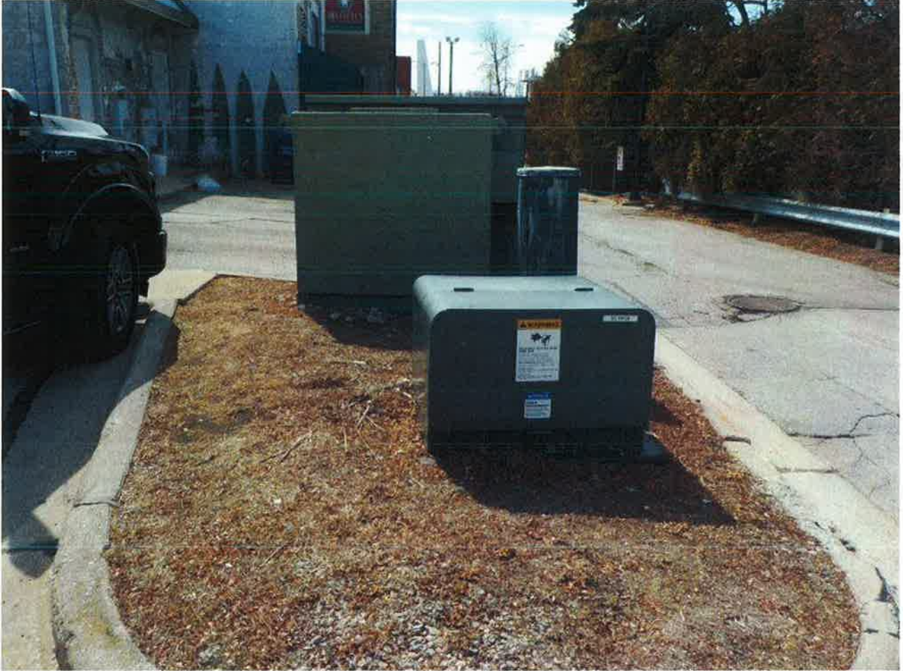
Transformers previously referenced.
