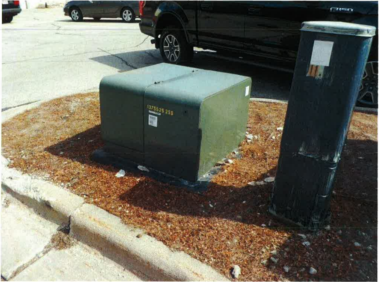
Pad mounted transformer along south property line.
