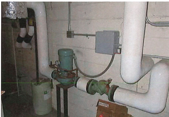
REHEAT COIL PUMP
