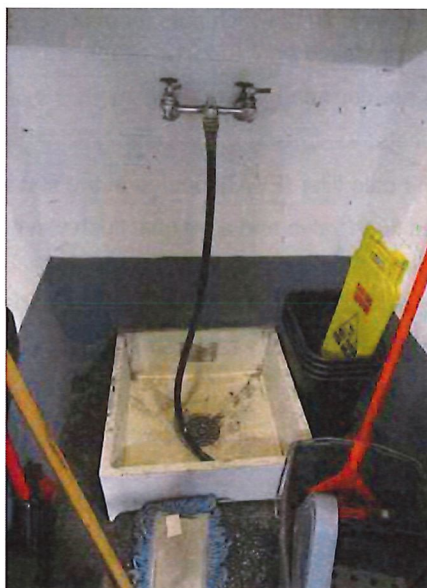
1ST FLOOR SERVICE SINK
