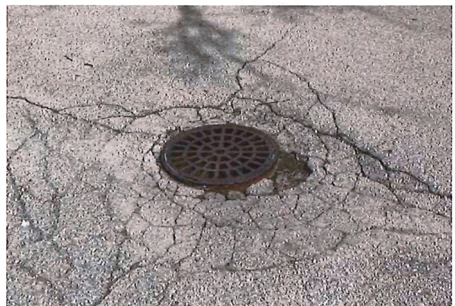
SITE PARKING LOT DRAIN
