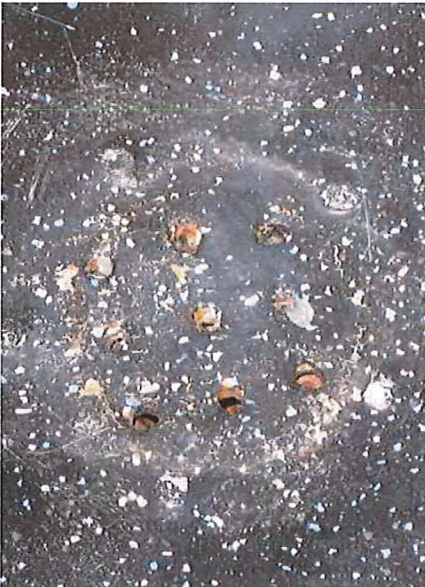
SHOWER ROOM FLOOR DRAIN GRATE
