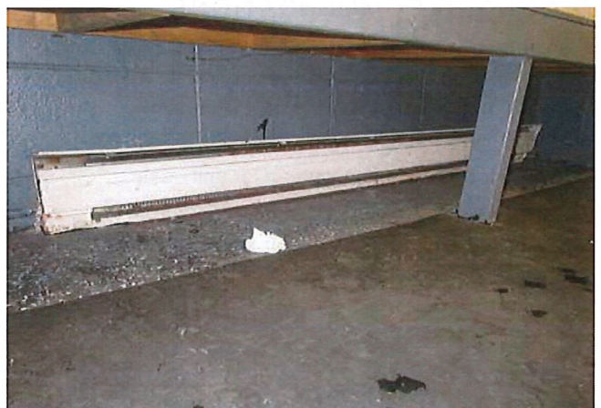
ELECTRIC BASEBOARD HEATER
