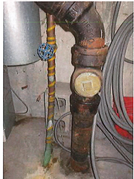
1 1/2" SUPPLY TO BELOW FLOOR – UNINSULATED/NOT LABELED AND HEAT TRACED
