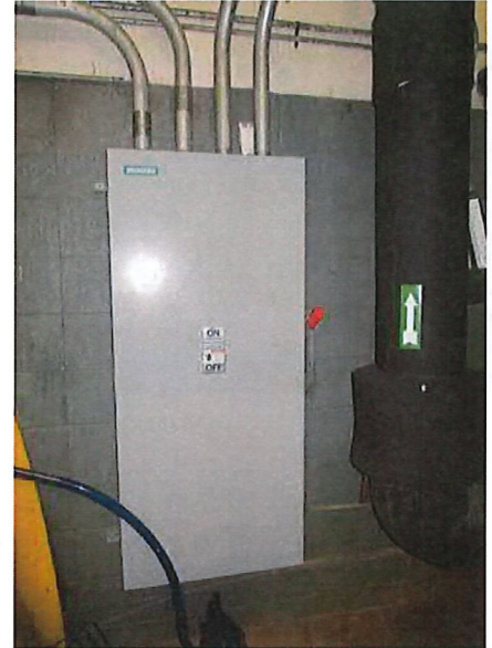
400 AMP MAIN DISCONNECT
