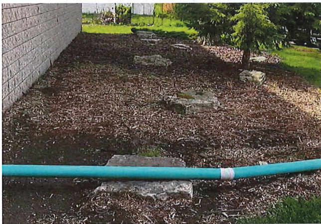
SURFACE ROOF DRAINAGE PIPE
