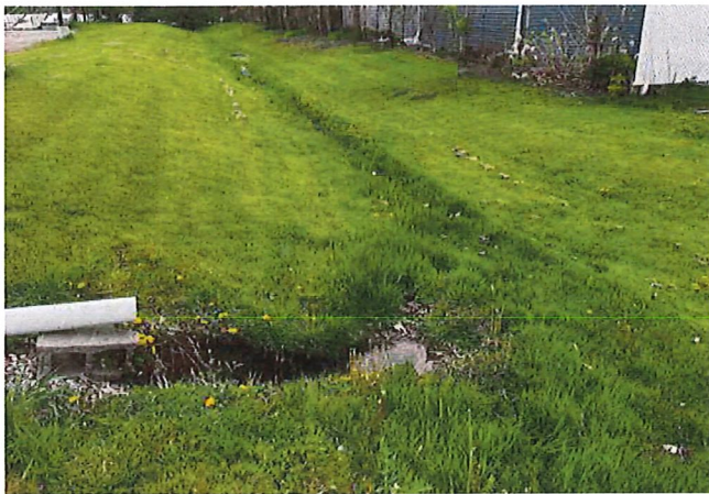
SOUTH DRAINAGE SWOLE
