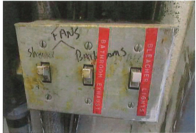
SHOWER AND RESTROOM FAN SWITCHES
