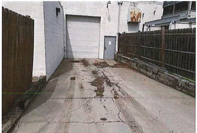
ZAMBONI ACCESS DOOR
