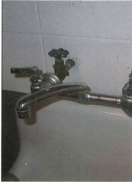
SERVICE SINK MISSING SUPPLY SHUT-OFF VALVE HANDLES AND VACUUM BREAKER
