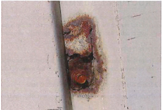
METAL SIDING CONNECTION RUSTED THROUGH
