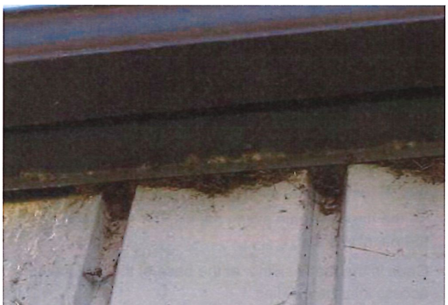
NEST IN SIDING GAPS UNDER THE ROOF GUTTERS
