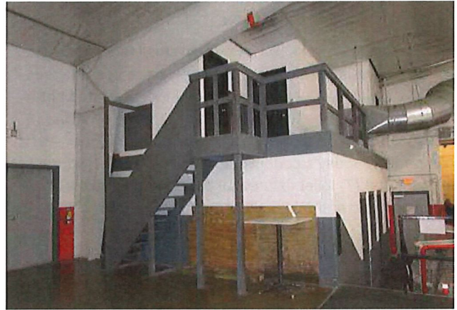
WOODEN STAIRS TO DEHUMIDIFIER EQUIPMENT
