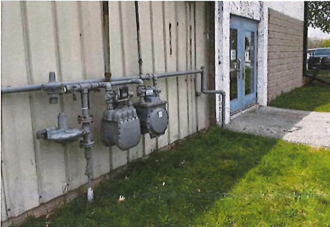
GAS SERVICE ENTRANCE
