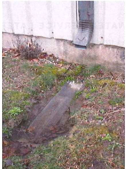
SEVERE PERIMETER GRADE EROSION
