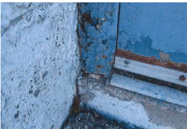
EXTERIOR METAL DOOR FRAME RUSTING
