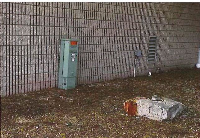
TELECOM BUILDING ENTRANCE
