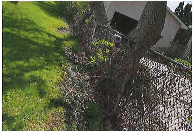
OVERGROWN TREES AT SOUTH PROPERTY LINE
