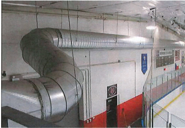
DEHUMIDIFICATION UNIT SUPPLY DUCTWORK
