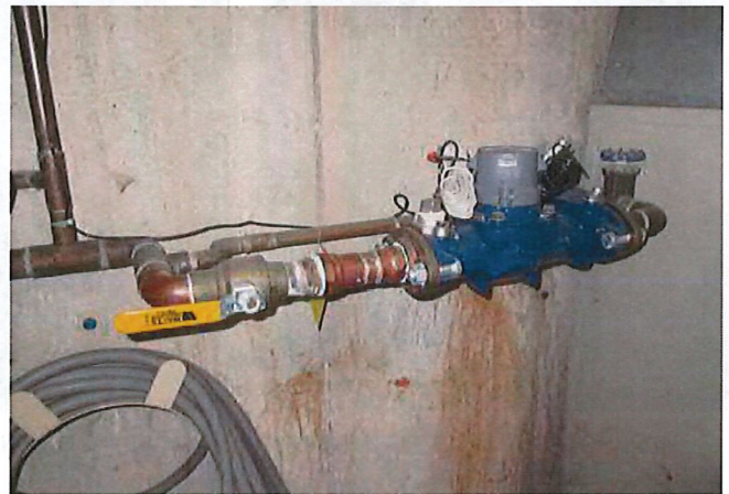
WATER SERVICE AND METER
