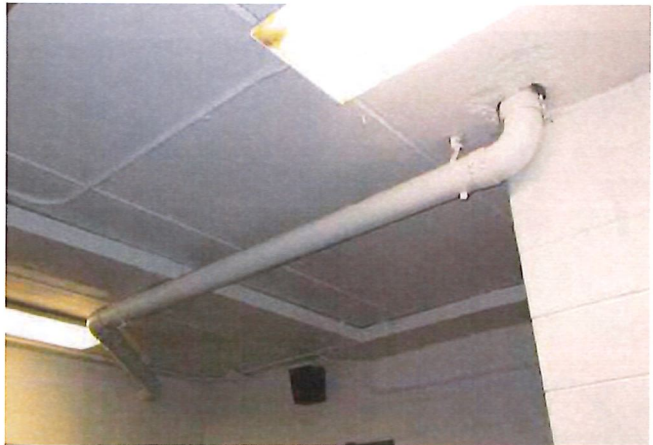
PAINTED CAST IRON PIPING
