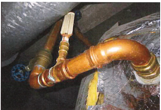
BROKEN THERMOMETER ON HOT WATER STORAGE TANK
