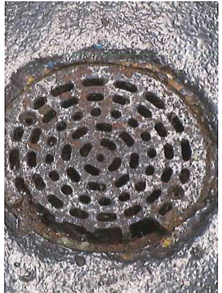
BROKEN FLOOR DRAIN GRATE
