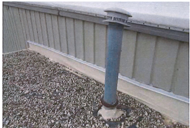
UNIT HEATER FLUE VENT
