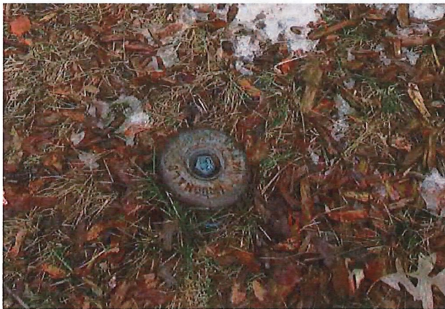
WATER SERVICE SHUT-OFF VALVE
