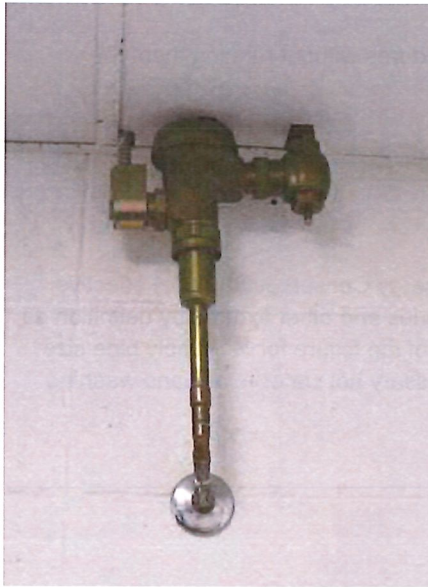
REMOTE URINAL FLUSH VALVE
