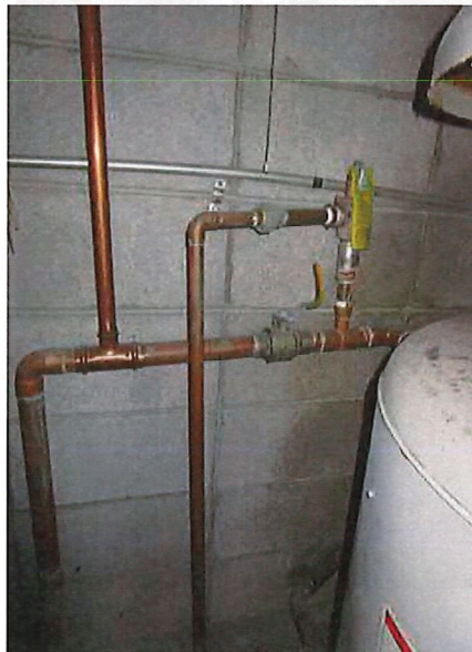
COPPER SUPPLY PIPING – NO INSULATION/NO LABELING
