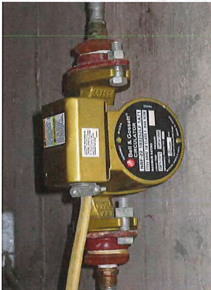
HOT WATER RECIRCULATING PUMP
