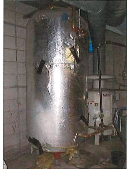
WATER HEATER/STORAGE TANK
