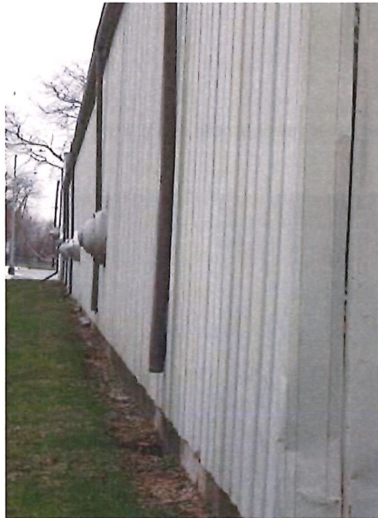
MISSING DOWNSPOUT EXTENSIONS
