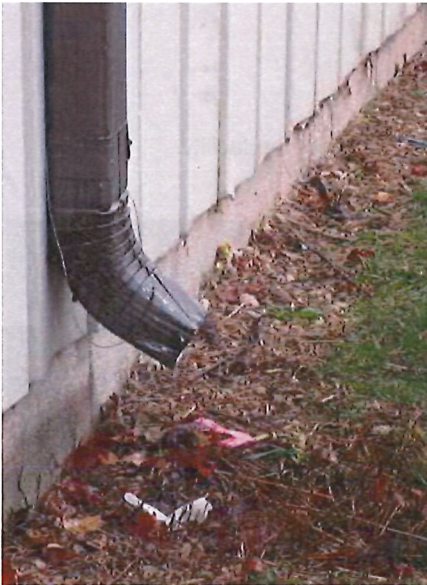
MISSING DOWNSPOUT EXTENSIONS
