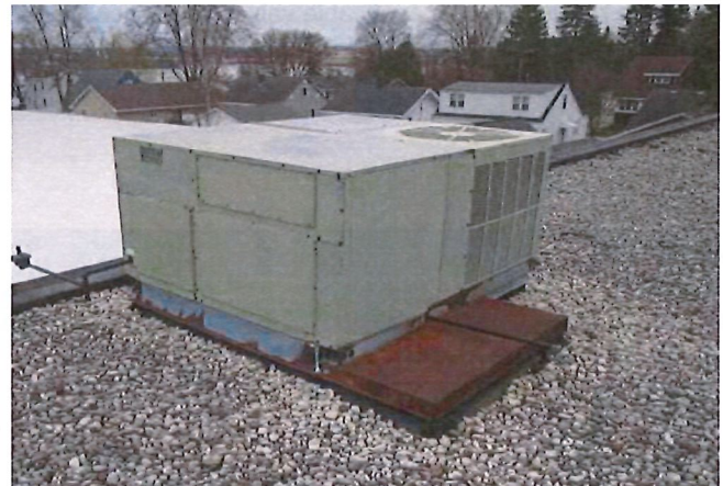
PACKAGED ROOFTOP UNIT
