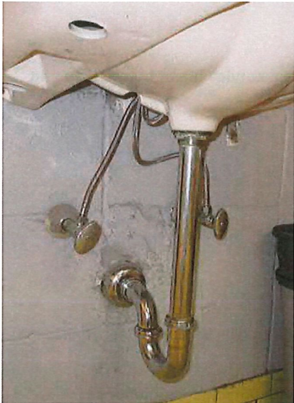
MISSING TRAP WRAP
