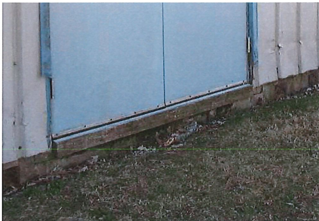
DROP OFF AT EXTERIOR EXIT DOOR
