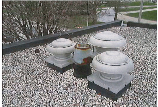
POWERED ROOF VENTILATORS AND COMMON FURNACE FLUE VENT
