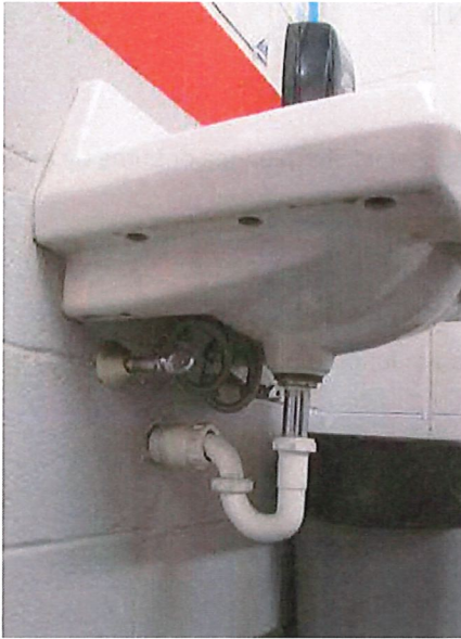
MISSING TRAP WRAP
