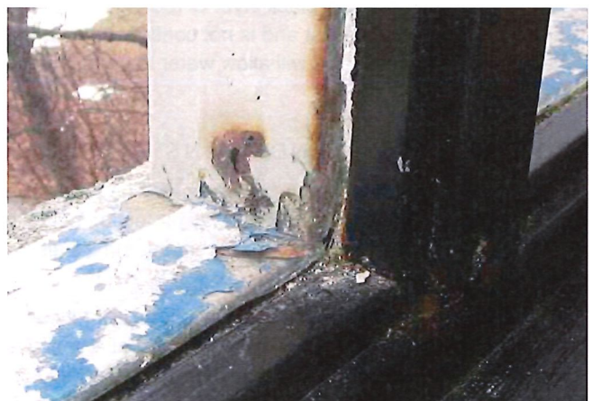
METAL WINDOW FRAME RUSTING FROM THE INSIDE
