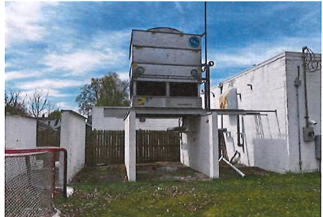
ICE EQUIPMENT CONDENSER
