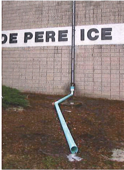
DOWNSPOUT PVC EXTENSION
