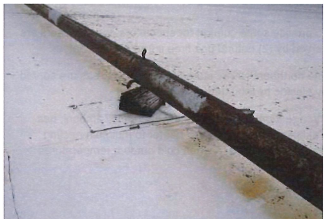
GAS PIPING ON ROOF
