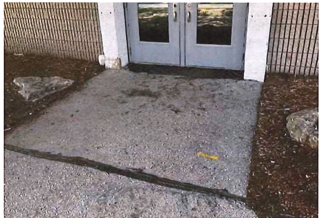
NO CONCRETE STOOP AT MAIN ENTRY
