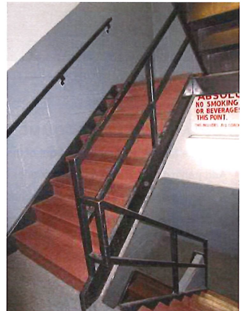
STAIR GUARD RAILS DO NOT MEET THE CURRENT CODE
