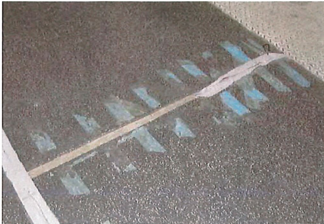
GAPS IN THE RUBBER FLOORING
