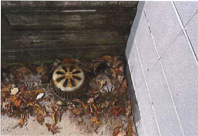
DEBRIS AT SURFACE DRAIN
