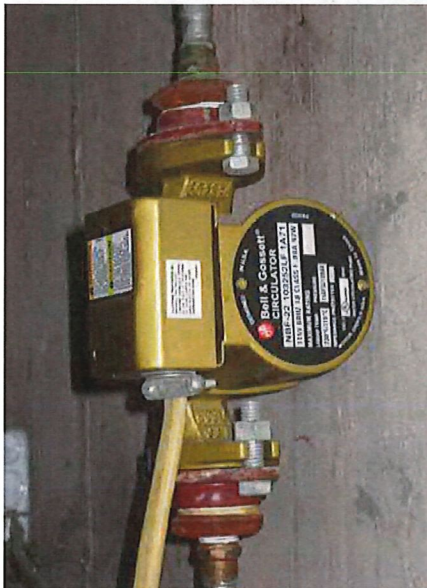
HOT WATER RECIRCULATING PUMP
