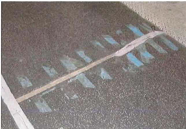
GAPS IN THE RUBBER FLOORING
