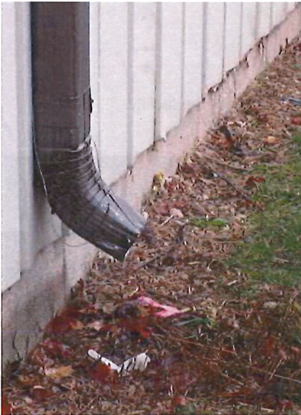
MISSING DOWNSPOUT EXTENSIONS
