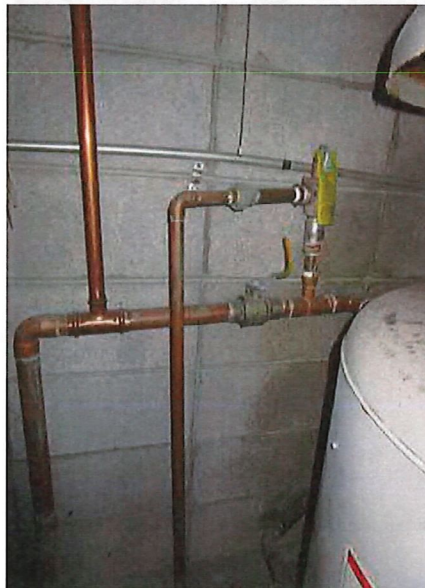
COPPER SUPPLY PIPING – NO INSULATION/NO LABELING
