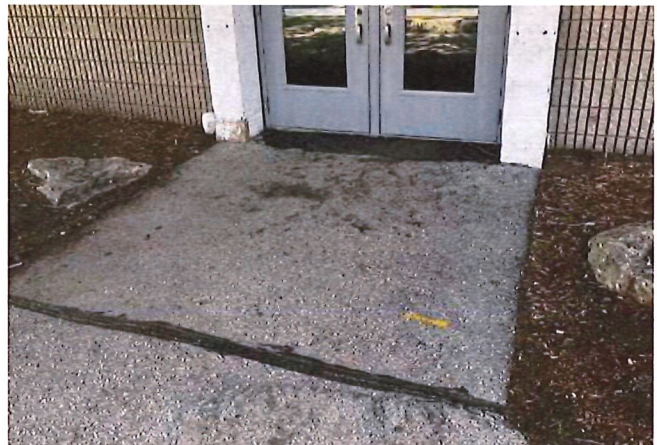
NO CONCRETE STOOP AT MAIN ENTRY
