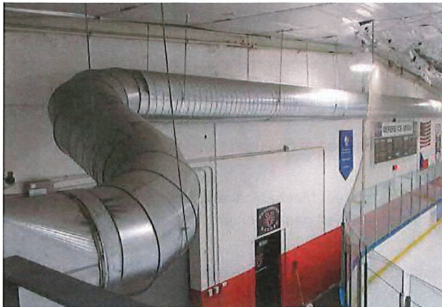
DEHUMIDIFICATION UNIT SUPPLY DUCTWORK
