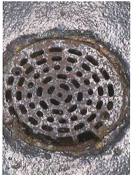
BROKEN FLOOR DRAIN GRATE
