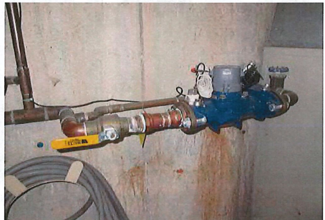
WATER SERVICE AND METER
