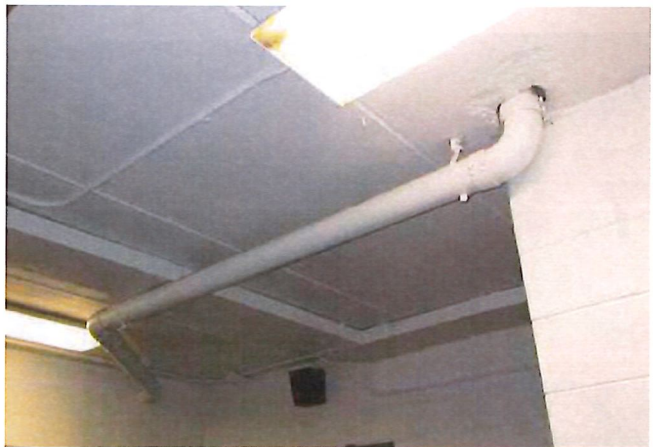
PAINTED CAST IRON PIPING
