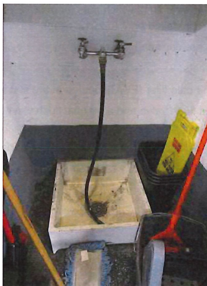
1ST FLOOR SERVICE SINK
