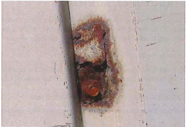
METAL SIDING CONNECTION RUSTED THROUGH
