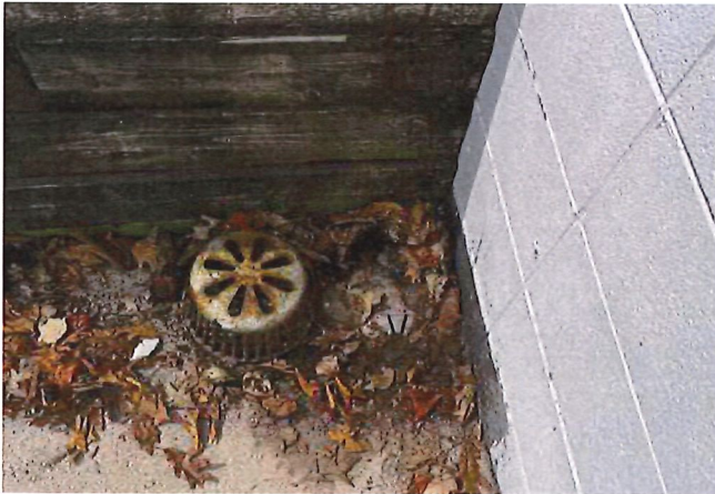
DEBRIS AT SURFACE DRAIN
