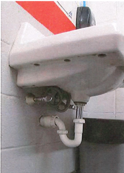
MISSING TRAP WRAP
