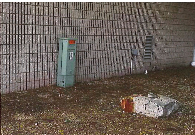
TELECOM BUILDING ENTRANCE
