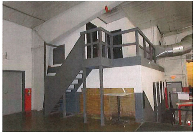
WOODEN STAIRS TO DEHUMIDIFIER EQUIPMENT
