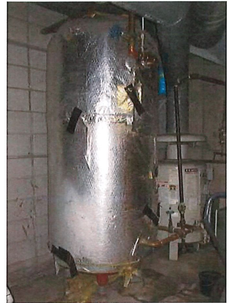
WATER HEATER/STORAGE TANK
