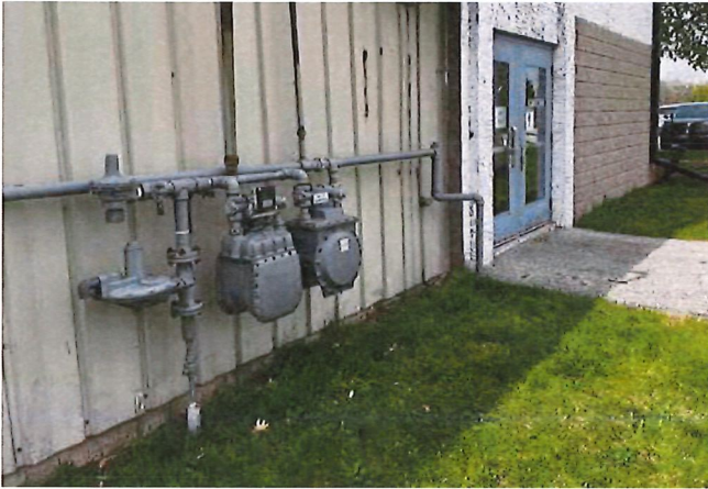
GAS SERVICE ENTRANCE
