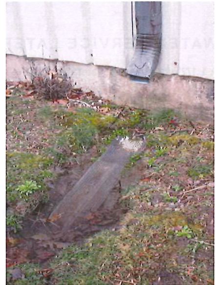
SEVERE PERIMETER GRADE EROSION
