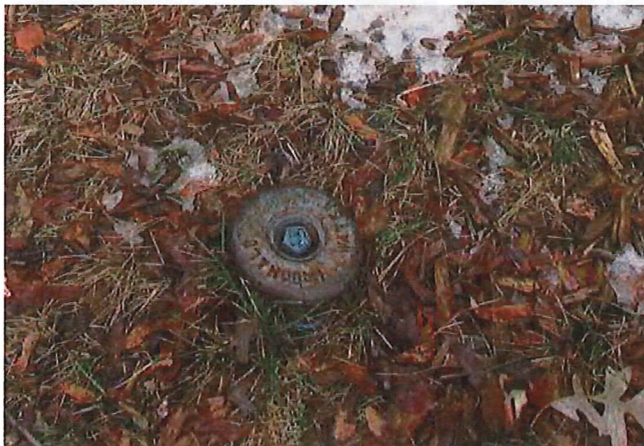
WATER SERVICE SHUT-OFF VALVE
