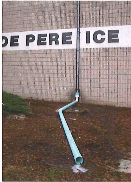
DOWNSPOUT PVC EXTENSION
