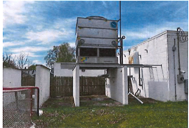
ICE EQUIPMENT CONDENSER
