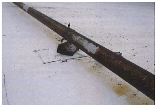
GAS PIPING ON ROOF
