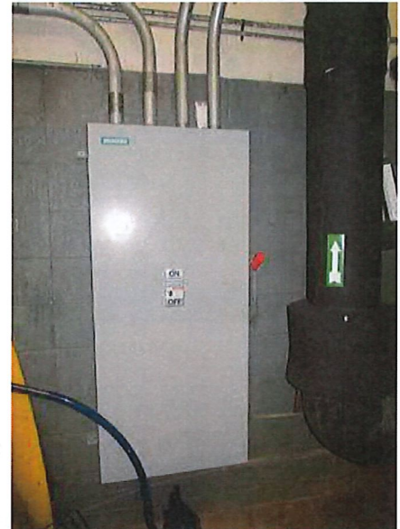
400 AMP MAIN DISCONNECT
