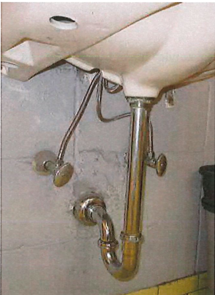
MISSING TRAP WRAP
