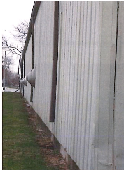
MISSING DOWNSPOUT EXTENSIONS
