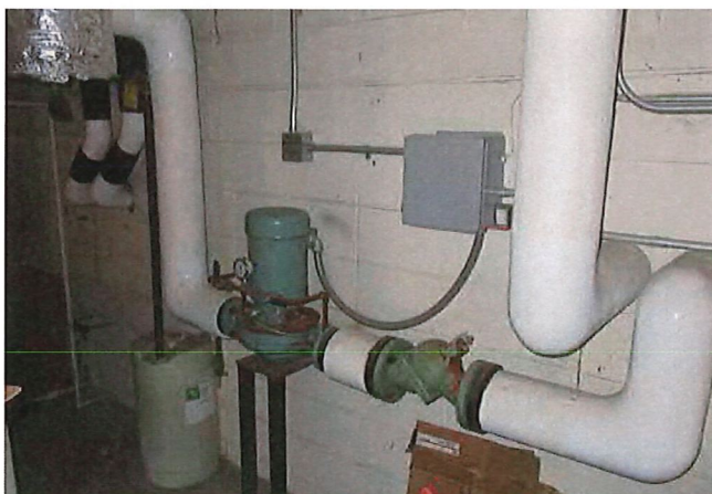
REHEAT COIL PUMP
