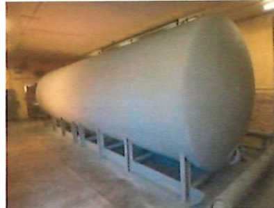
Iron Manganese Filter tank
