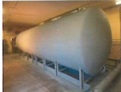
Iron Manganese Filter tank
