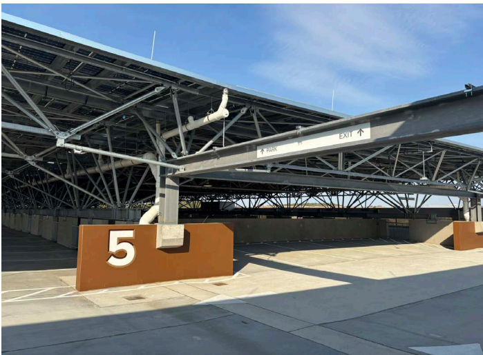
Photovoltaic Panel Framing - UW Health EastHub Parking Structure
