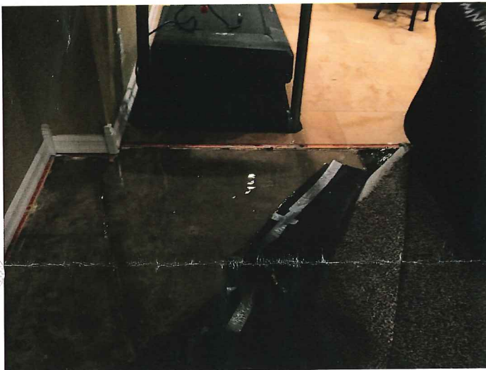
This is one of our carpeted areas in our basement completely drenched as it soaked up the 1.5"-2" of water.
