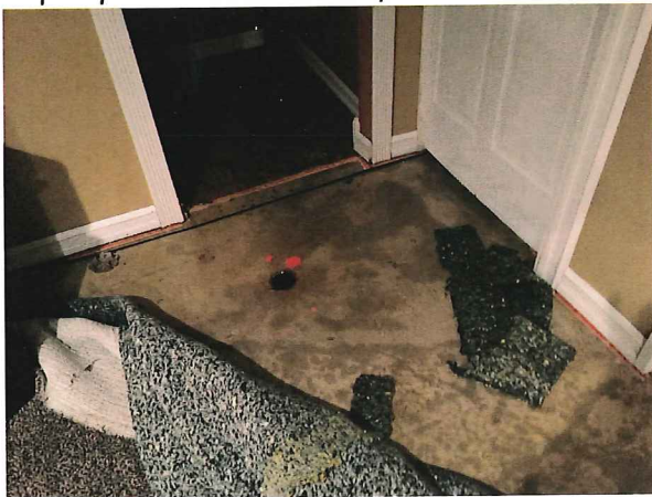
This is difficult to see, but the water is swirling down the drain located beneath our carpet and leading into our bathroom area.
