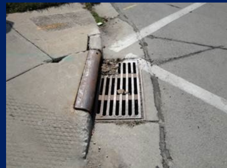
Above: Parallel drainage grate
