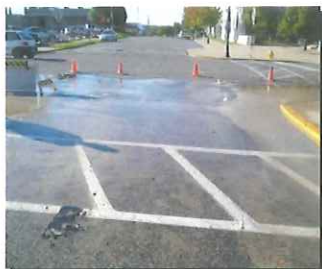
Leak surfacing at intersection
