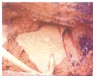
Hidden leak running into drain tile
