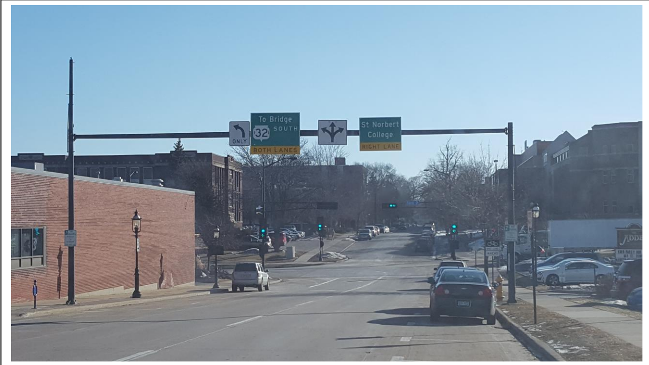
Overhead Street pole with broken banner support pole
