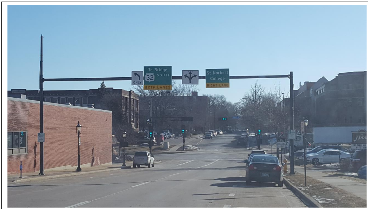
Overhead Street pole with broken banner support pole
