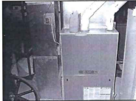
Basement area furnace
