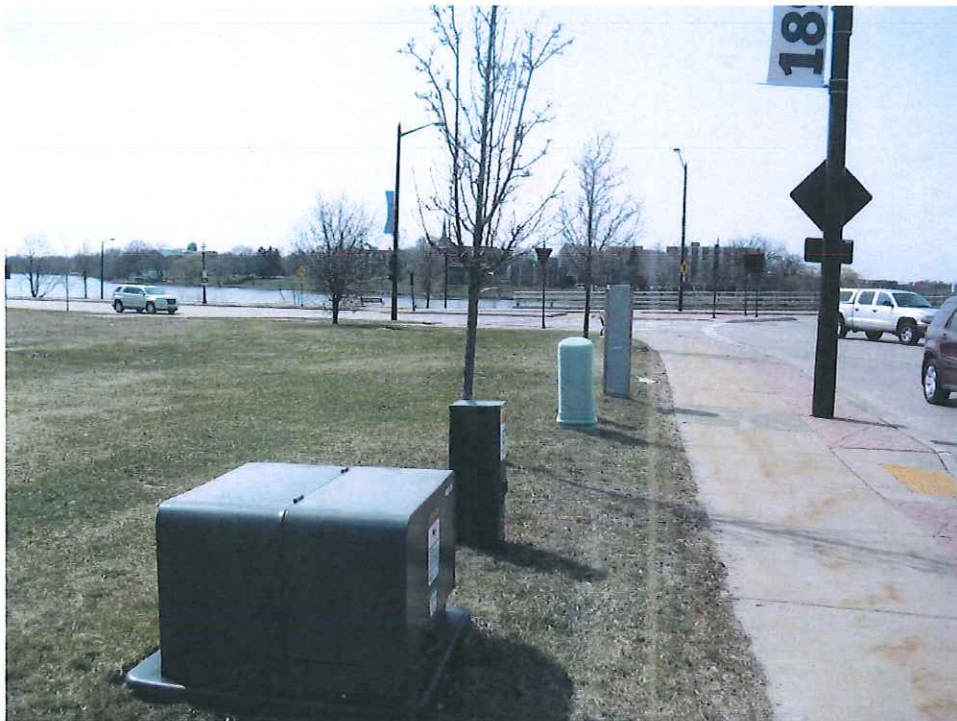
Historic Parcel ED-814 facing southwest, showing transformer and cable boxes
