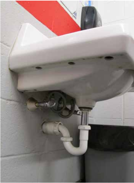
MISSING TRAP WRAP
