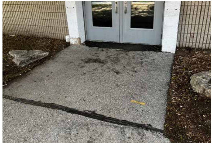
NO CONCRETE STOOP AT MAIN ENTRY
