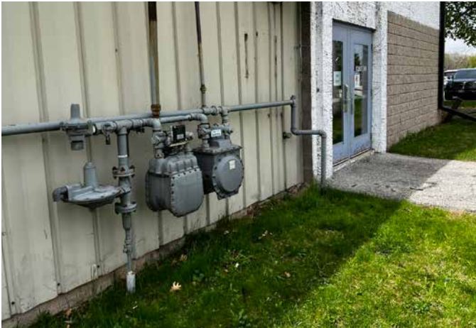
GAS SERVICE ENTRANCE
