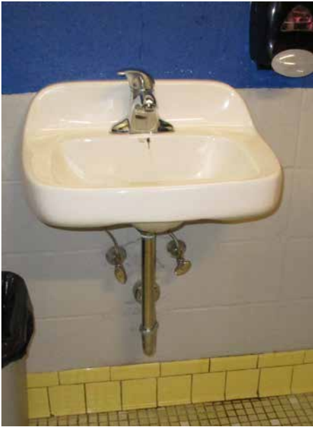
MISSING TRAP WRAP
