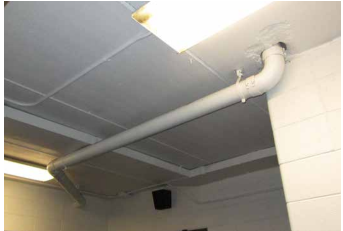
PAINTED CAST IRON PIPING
