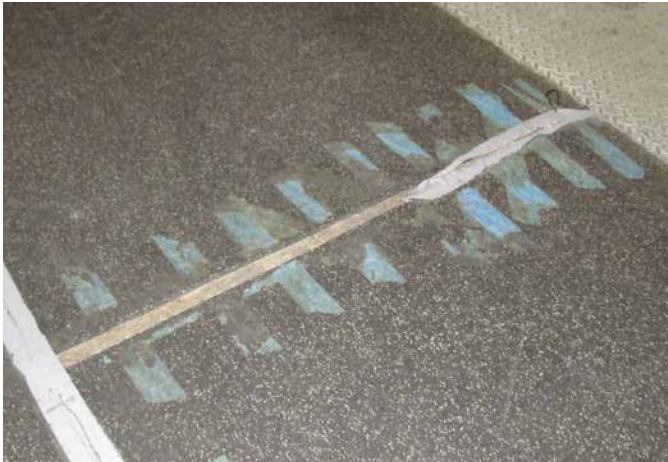
GAPS IN THE RUBBER FLOORING
