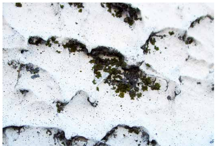
LICHEN GROWING ON BUILDING FACE
