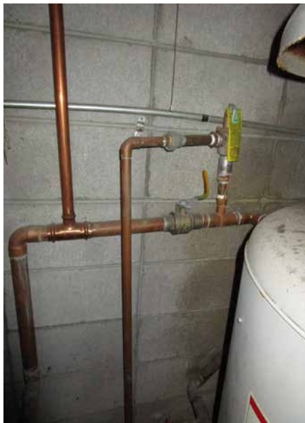
COPPER SUPPLY PIPING – NO INSULATION/NO LABELING
