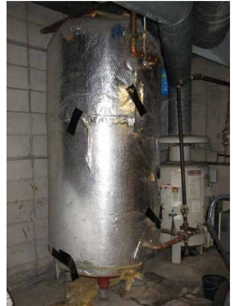
WATER HEATER/STORAGE TANK
