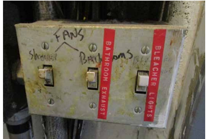
SHOWER AND RESTROOM FAN SWITCHES
