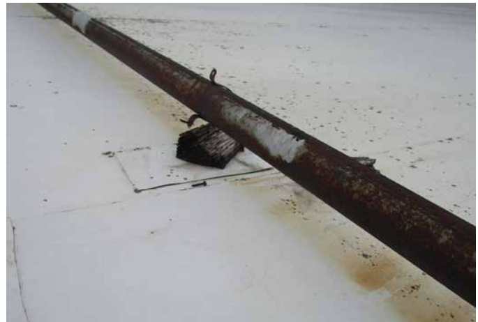
GAS PIPING ON ROOF
