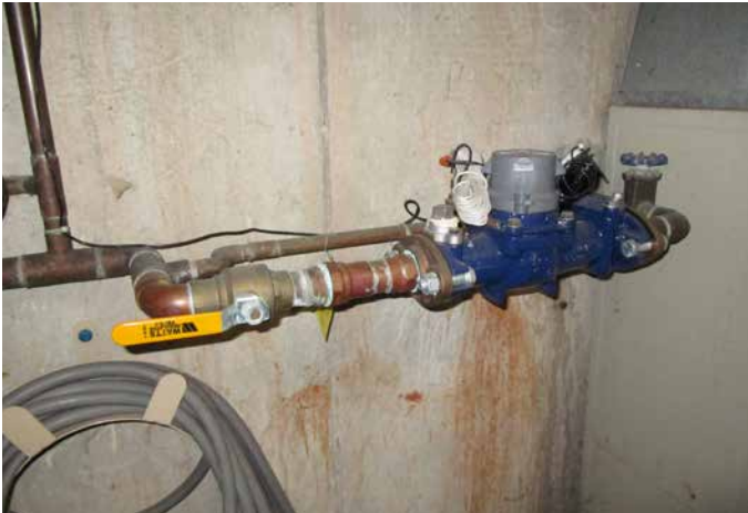
WATER SERVICE AND METER
