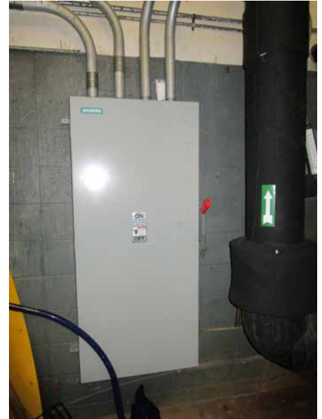
400 AMP MAIN DISCONNECT
