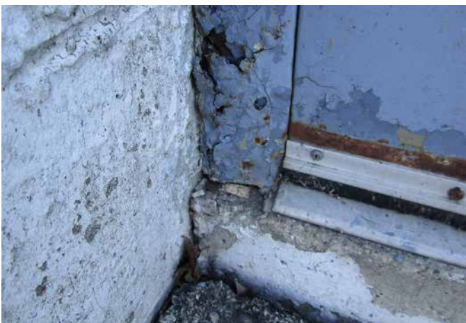
EXTERIOR METAL DOOR FRAME RUSTING
