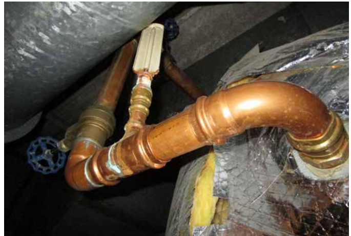
BROKEN THERMOMETER ON HOT WATER STORAGE TANK
