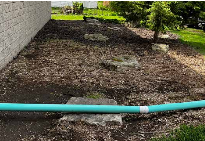
SURFACE ROOF DRAINAGE PIPE
