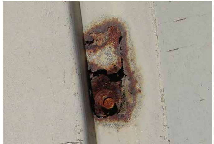
METAL SIDING CONNECTION RUSTED THROUGH
