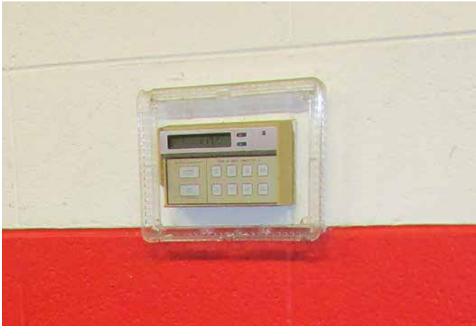
BASEMENT LOCKERS PROGRAMMABLE THERMOSTAT
