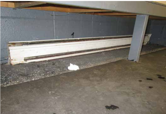
ELECTRIC BASEBOARD HEATER
