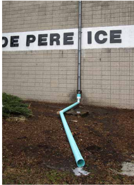
DOWNSPOUT PVC EXTENSION
