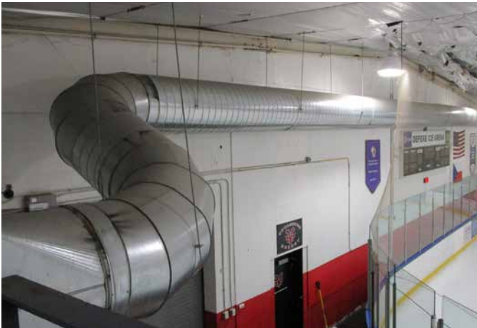
DEHUMIDIFICATION UNIT SUPPLY DUCTWORK
