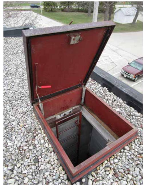
ROOF HATCH INSTALLED BACKWARDS
