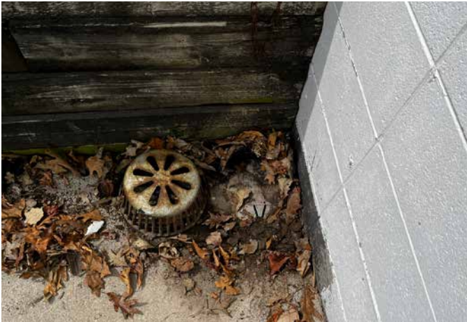
DEBRIS AT SURFACE DRAIN
