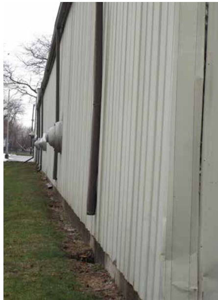
MISSING DOWNSPOUT EXTENSIONS
