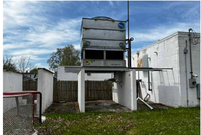
ICE EQUIPMENT CONDENSER
