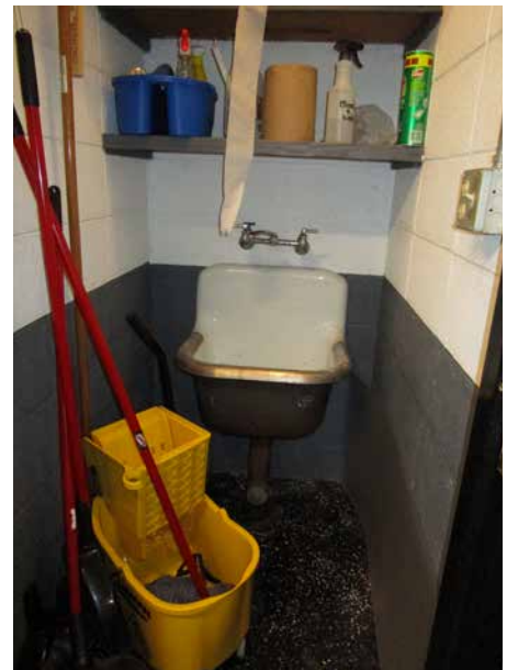
2ND FLOOR SERVICE SINK
