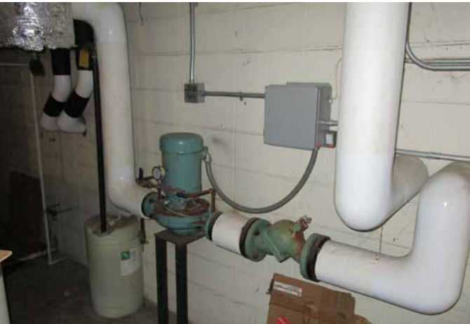
REHEAT COIL PUMP
