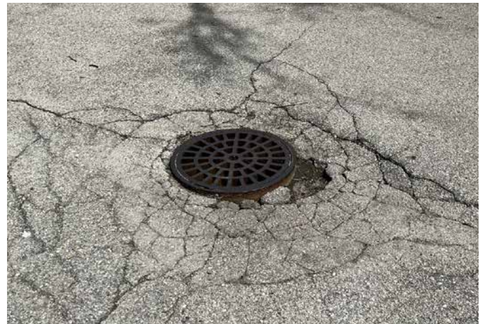
SITE PARKING LOT DRAIN
