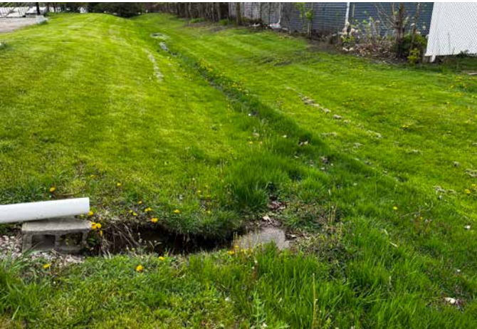
SOUTH DRAINAGE SWOLE
