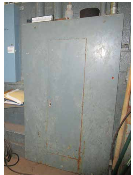
MAIN DISTRIBUTION PANEL
