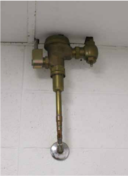
REMOTE URINAL FLUSH VALVE
