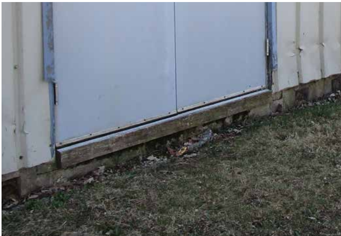
DROP OFF AT EXTERIOR EXIT DOOR
