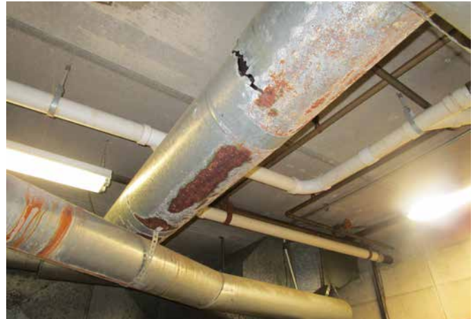
DETERIORATED FLUE VENTING FOR FURNACE #1 AND #2
