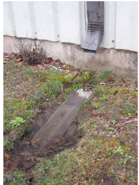
SEVERE PERIMETER GRADE EROSION
