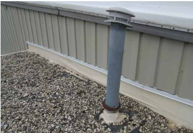
UNIT HEATER FLUE VENT
