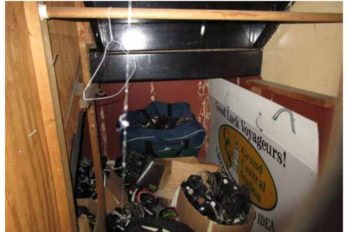
STORAGE UNDER EXIT STAIRWAYS
