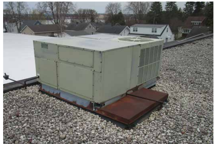
PACKAGED ROOFTOP UNIT
