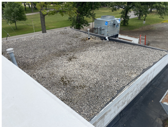
Looking down on the failing roof
