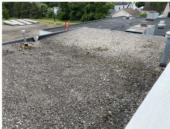
Looking down on the failing roof
