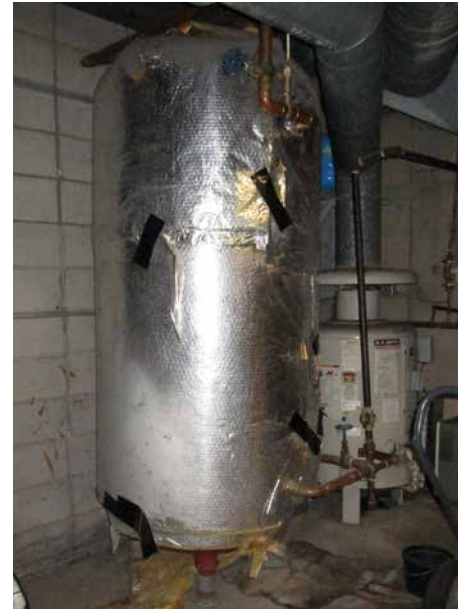
WATER HEATER/STORAGE TANK
