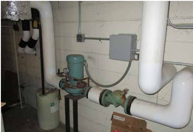
REHEAT COIL PUMP
