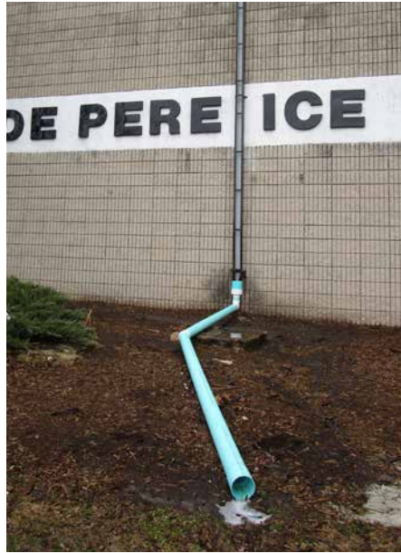
DOWNSPOUT PVC EXTENSION
