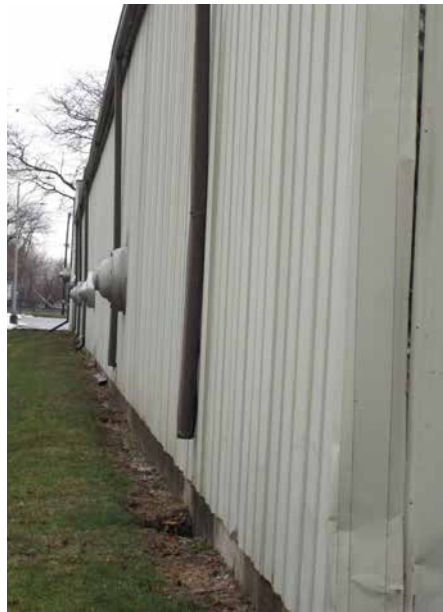
MISSING DOWNSPOUT EXTENSIONS
