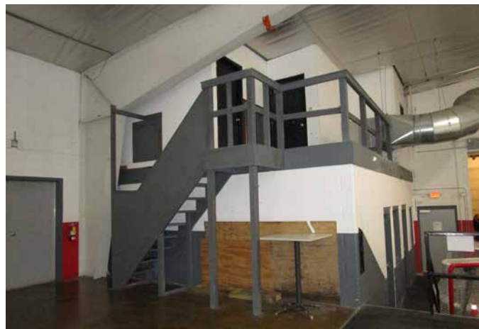
WOODEN STAIRS TO DEHUMIDIFIER EQUIPMENT
