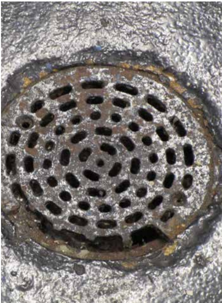
BROKEN FLOOR DRAIN GRATE
