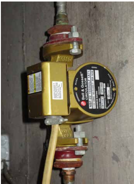
HOT WATER RECIRCULATING PUMP
