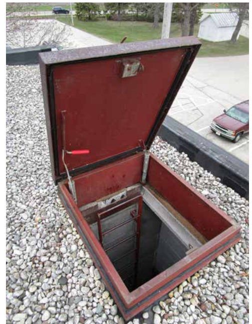
ROOF HATCH INSTALLED BACKWARDS
