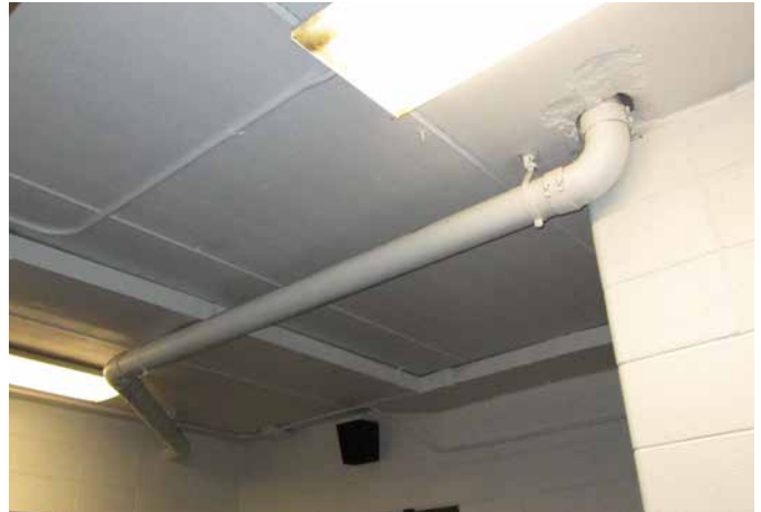
PAINTED CAST IRON PIPING
