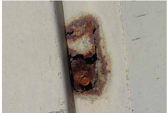
METAL SIDING CONNECTION RUSTED THROUGH
