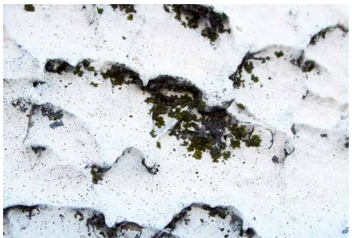
LICHEN GROWING ON BUILDING FACE
