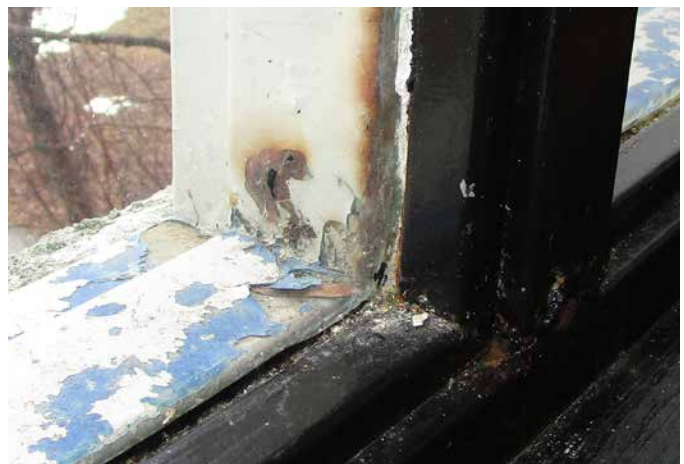
METAL WINDOW FRAME RUSTING FROM THE INSIDE
