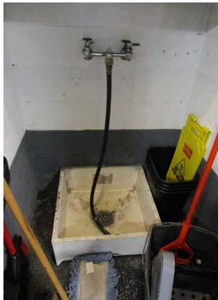
1ST FLOOR SERVICE SINK
