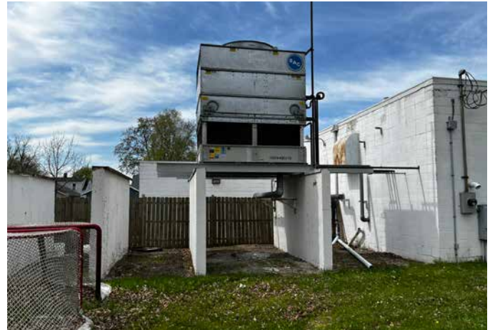
ICE EQUIPMENT CONDENSER
