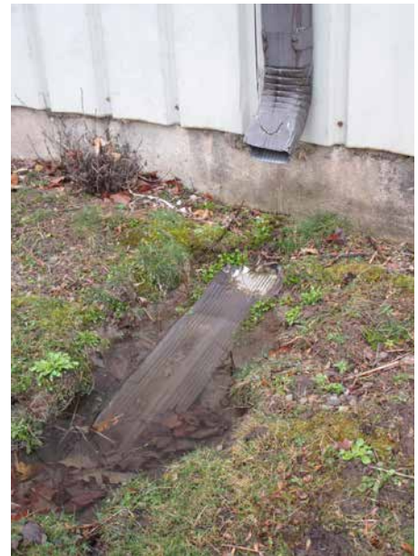
SEVERE PERIMETER GRADE EROSION
