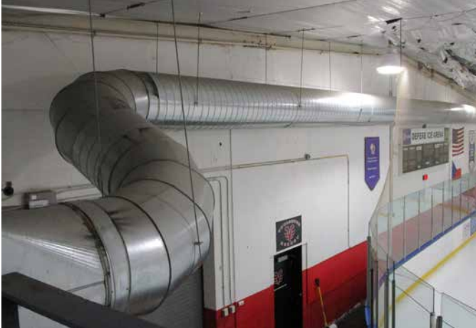
DEHUMIDIFICATION UNIT SUPPLY DUCTWORK
