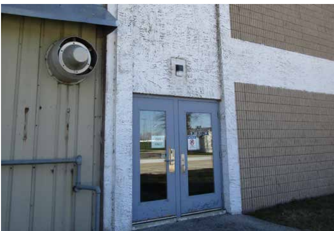
TEXTURED STUCCO HOLDING DIRT
