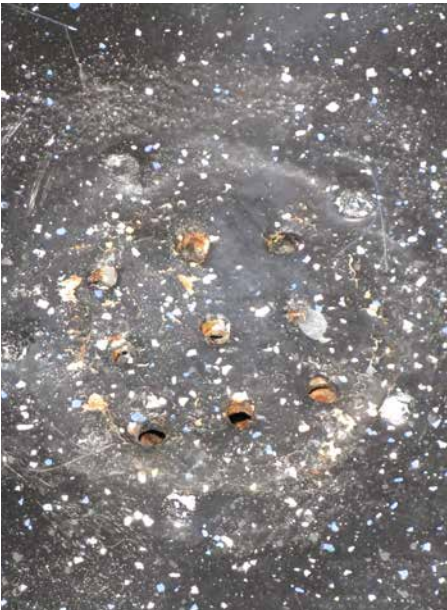
SHOWER ROOM FLOOR DRAIN GRATE
