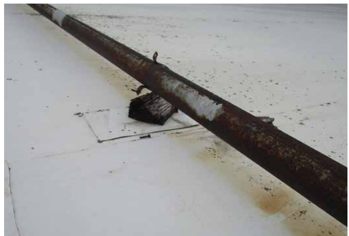
GAS PIPING ON ROOF
