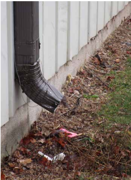
MISSING DOWNSPOUT EXTENSIONS
