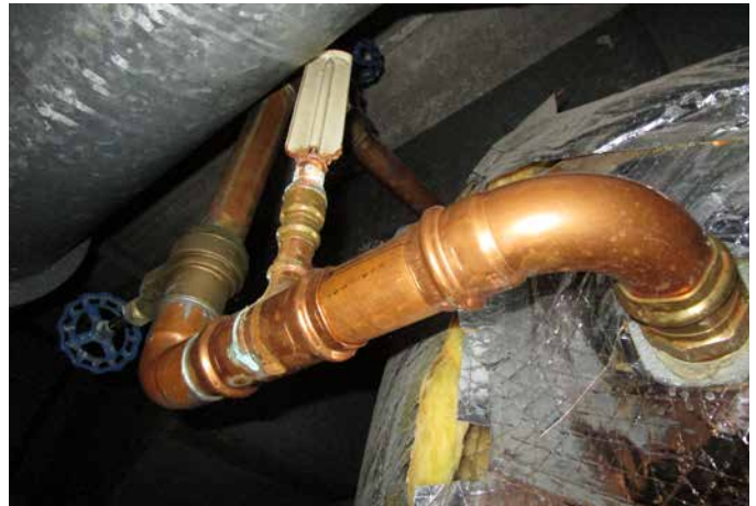
BROKEN THERMOMETER ON HOT WATER STORAGE TANK
