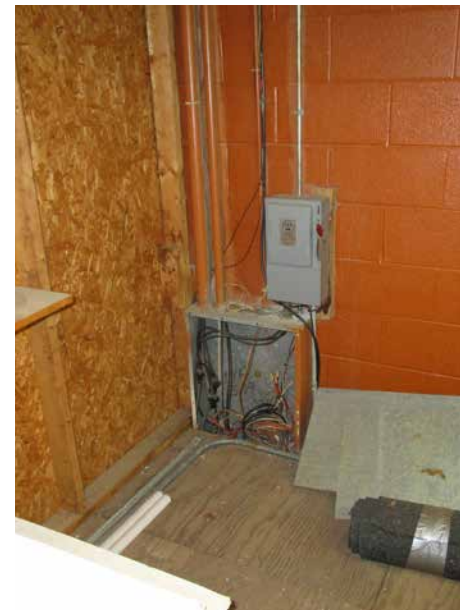
OPEN JUNCTION BOX
