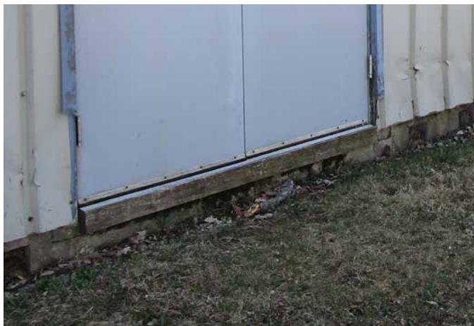
DROP OFF AT EXTERIOR EXIT DOOR
