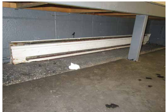
ELECTRIC BASEBOARD HEATER
