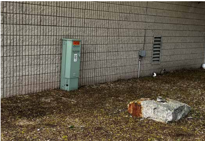
TELECOM BUILDING ENTRANCE
