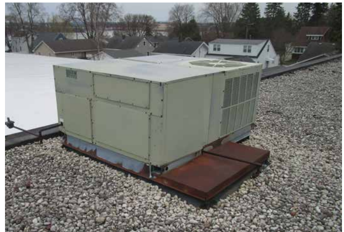
PACKAGED ROOFTOP UNIT
