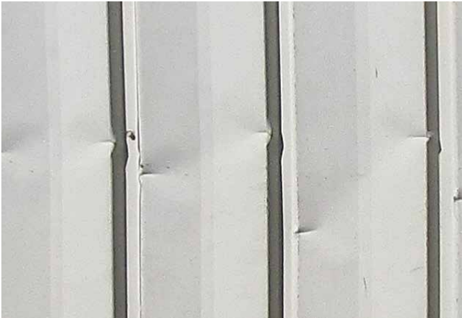
CRIMPED METAL SIDING AT ARENA BASE
