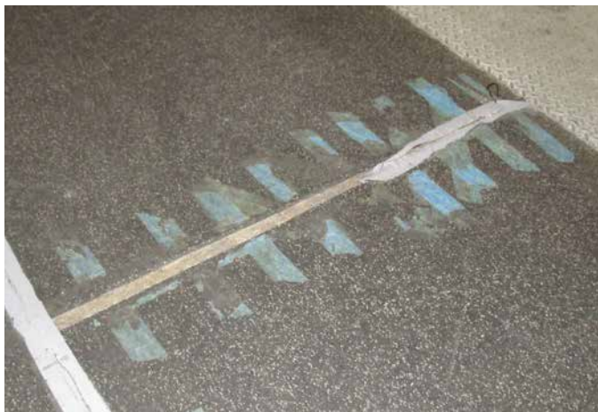
GAPS IN THE RUBBER FLOORING
