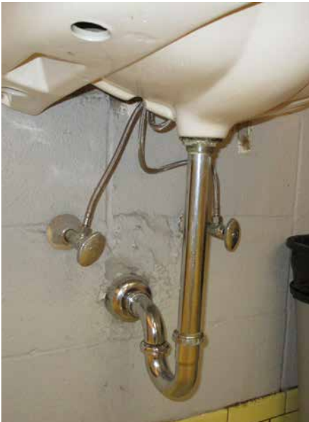
MISSING TRAP WRAP
