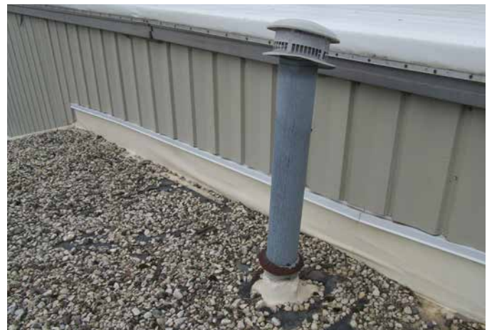
UNIT HEATER FLUE VENT
