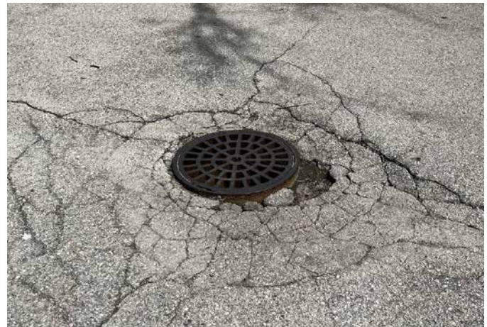
SITE PARKING LOT DRAIN
