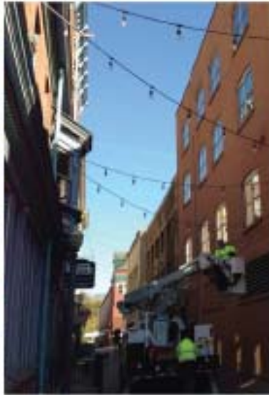
1G - Alley Lighting
