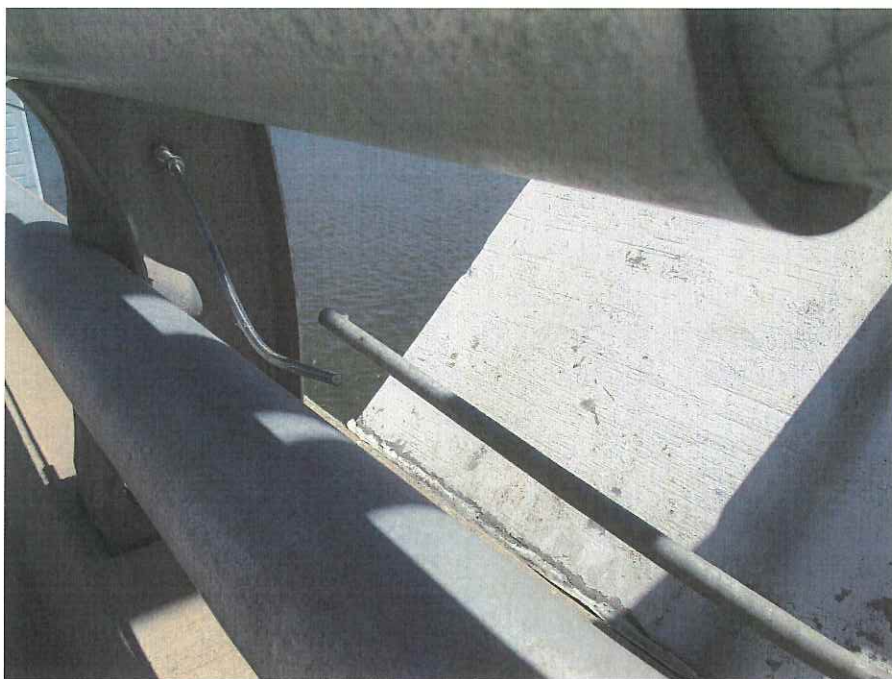
Figure 3. South side, sixth pier from West snapped cable
